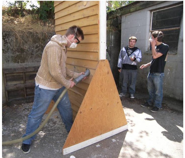
The Building Performance Center's Weatherization Technology workshop was one of the "green" activities
